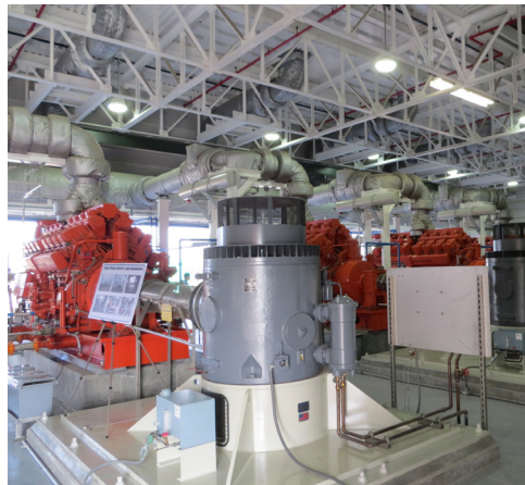
OCPW - Los Alamitos Stormwater Pump Station
