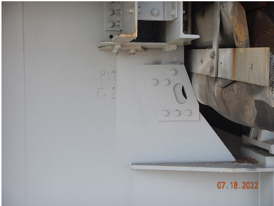
Figure 8. Final typical repair at web reprofiling (plate on opposite side not visible). (Courtesy of IDOT)
